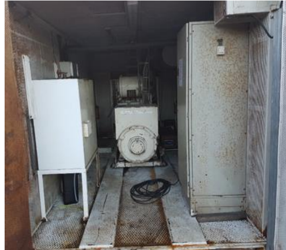
Cummins KTA-1150-G2 400/500 KVA Generator
